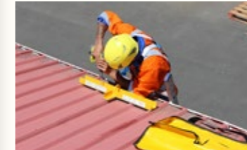
Anchor Point using Temporary Roof Anchor
